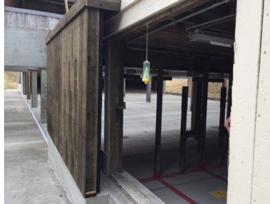
Armored steel side wall
