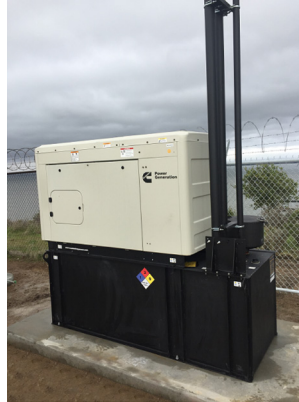
New emergency generator
