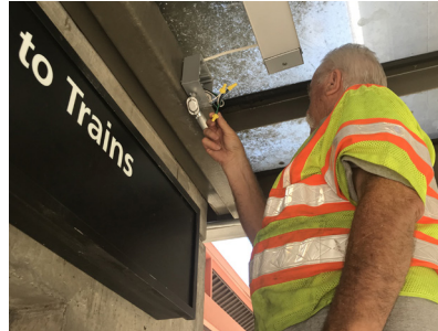
New light installation
