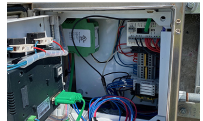
Integrated flow rate/leak detection system
