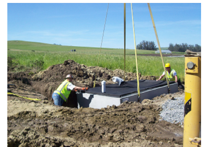
Filterra system placement
