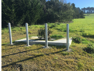
Operational Filterra unit
