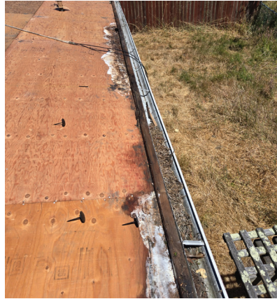
Roof Deck to be Replaced
