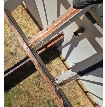
Roof Framing to be Replaced
