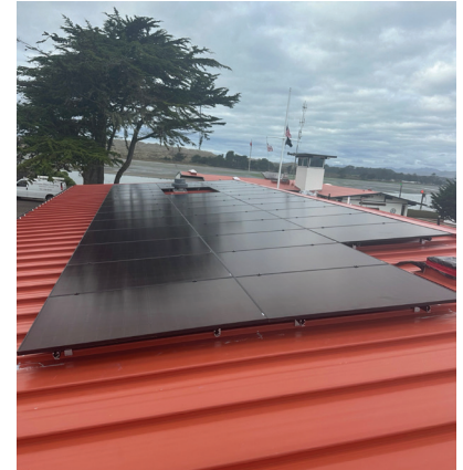
UPH Solar Array & New Metal Roof
