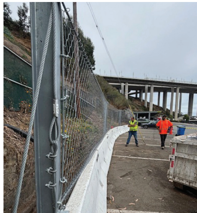
New T35 Rockfall Barrier
